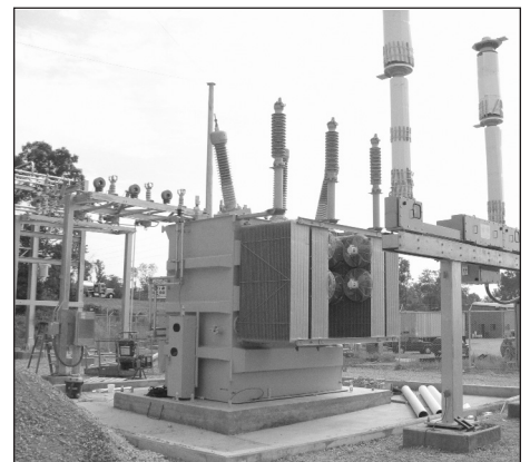
The substation also features the most up-to-date environmental safety features. Each of the transformers is mounted on a concrete pad with a built-in drainage system that will divert any accidental oil spill to a holding tank for proper disposal.
