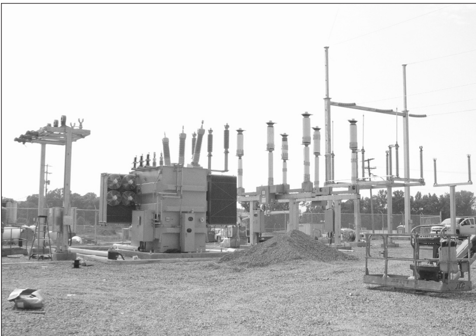
This photo taken during construction features one of the two 25MVA transformers that are the core of the new "Tennol" substation.
